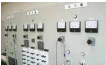
▲ The power Transmission Systems Simulator
