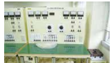
▲ Experimental Equipment for Electromechanical Systems & Power Electronics
